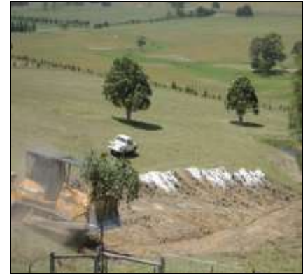
Department of Lands undertaking remedial works on gully 1, which feeds into the farms main dam for livestock.
